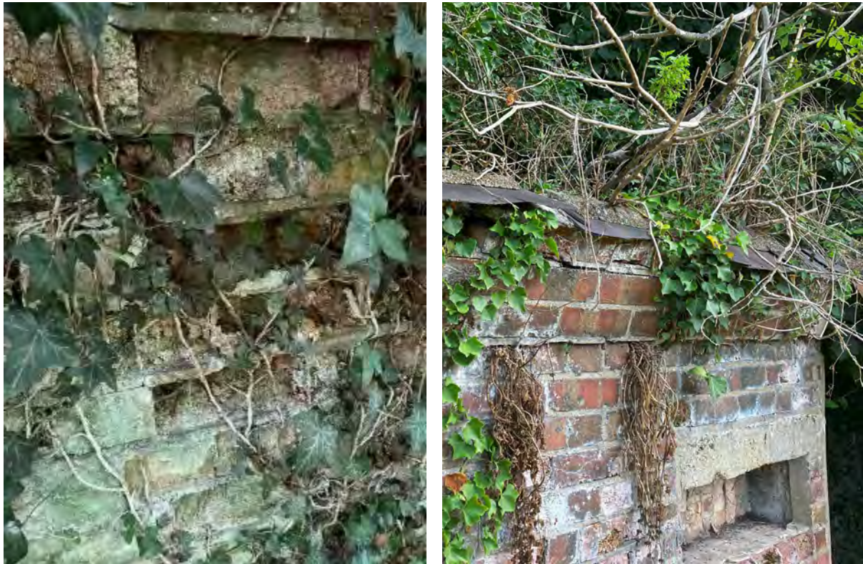
Figure 16: Pillbox 2 brickwork damage (Monument ID 6)
