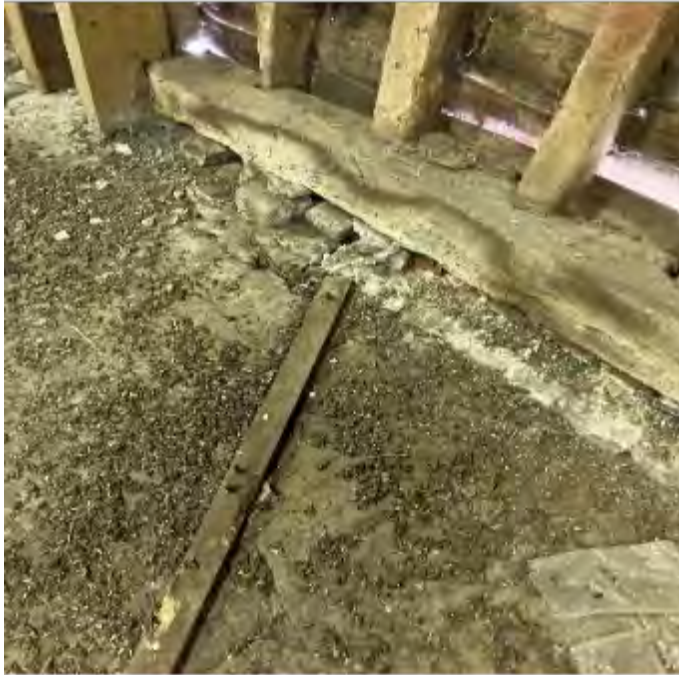
Figure 4: Deteriorating sole plate
