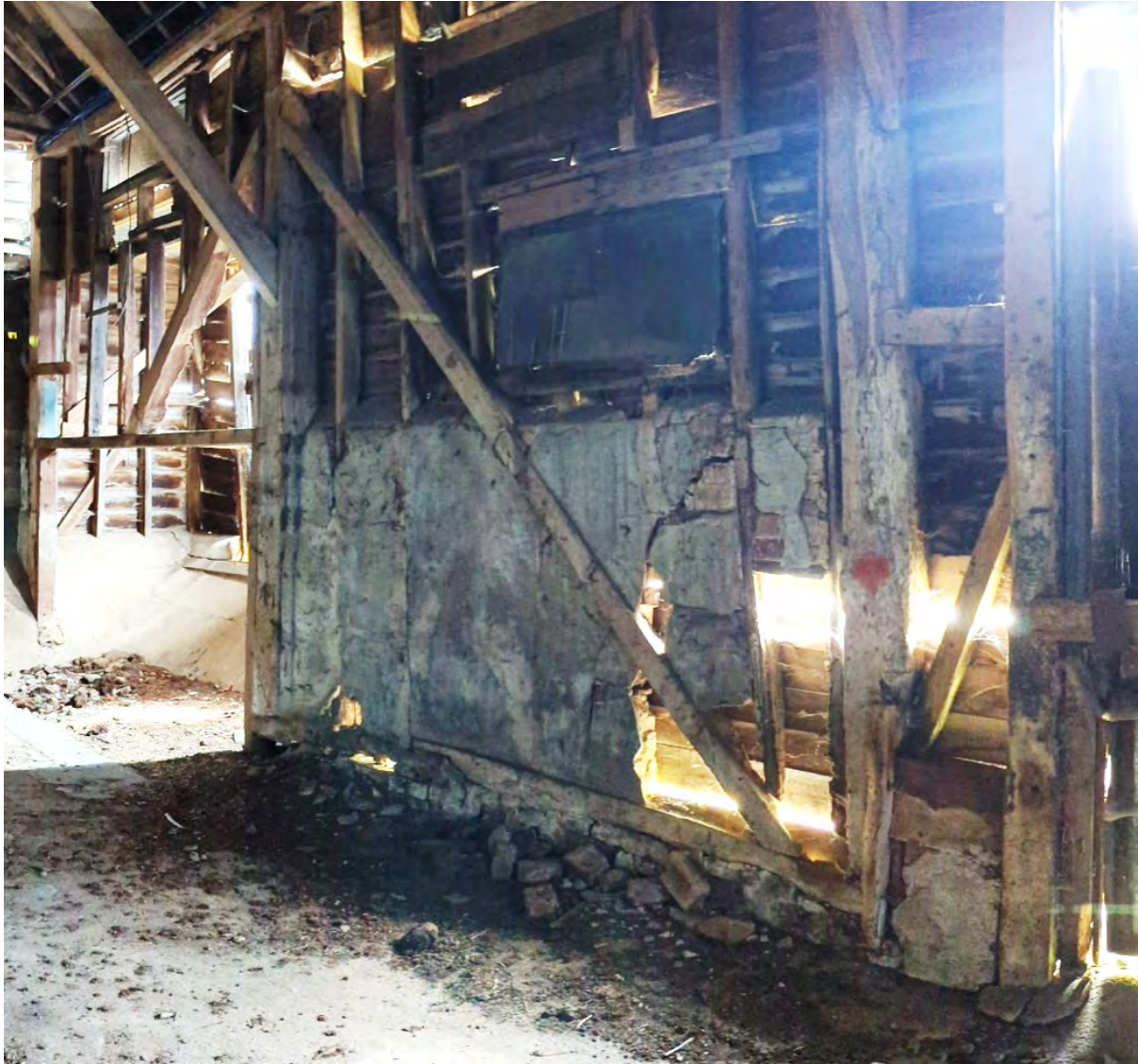
Figure 10: South barn material deterioration
