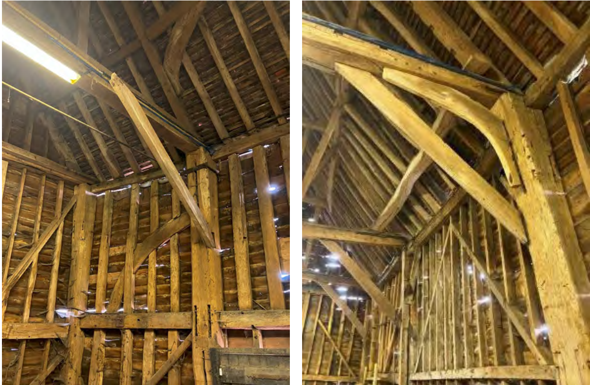
Figure 3: Black Barn northern diagonal additional braces
