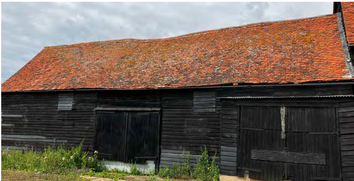
Figure 8: South barn sagging roof
